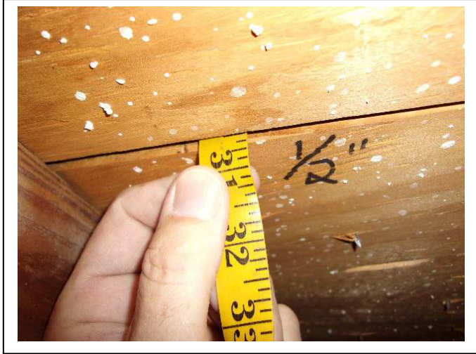
ROOF DECK THICKNESS – 15/32 to 1/2 inch plywood
